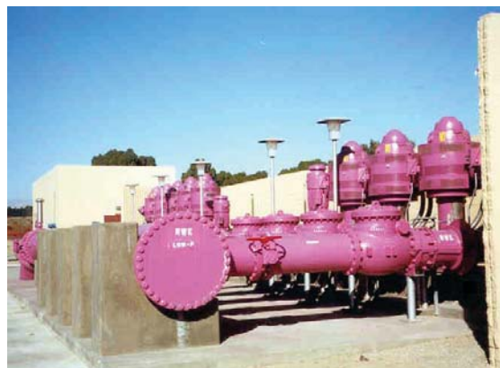
CVWD Recycled Water Pump Station
