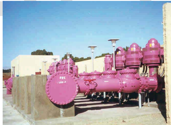
CVWD Recycled Water Pump Station
