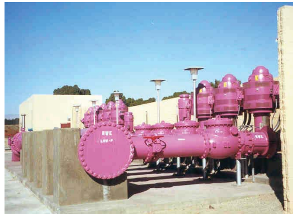
CVWD Recycled Water Pump Station
