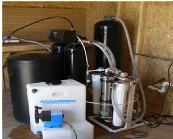
Example of a reverse osmosis system installed in the San Antonio del Desierto Mobile Home Park by Pueblo Unido Community Development Corporation for the STAT Project.
