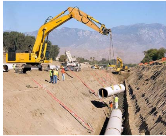
Mid-Valley Pipeline, the backbone of CVWD’s Non-Potable Water System Source: CVWD 2010
