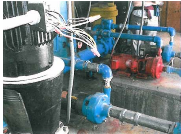
Uncovered electrical boxes at pumping station. Other electrical issues contributed to pump failures, including failure of fire pump.
