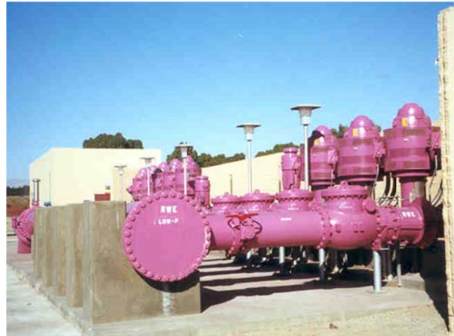
CVWD Recycled Water Pump Station
